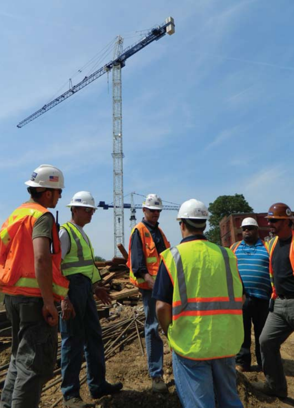
Members of the Clark field engineering team (in orange vests) and Leica representative Bill Murphy explain the workings of the monitoring system to PSM editor, TJ Frazier (foreground).
