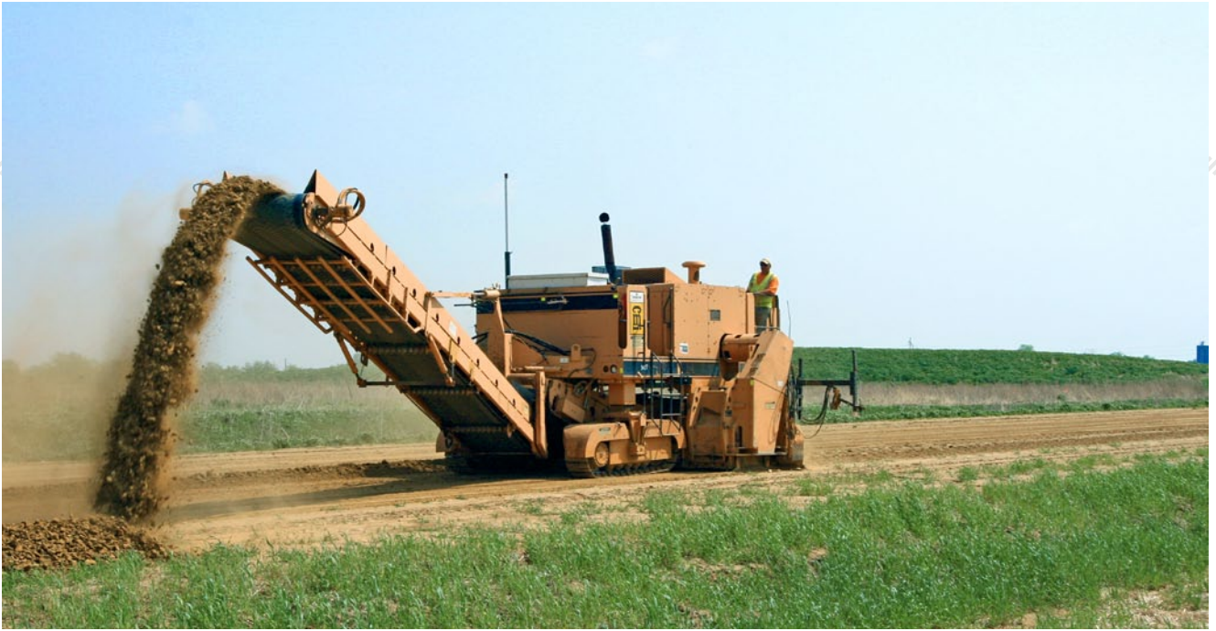
A CMI trimmer—equipped with a PowerGrade 3D controls from Leica Geosystems—trimmed the dirt precisely to grade.
