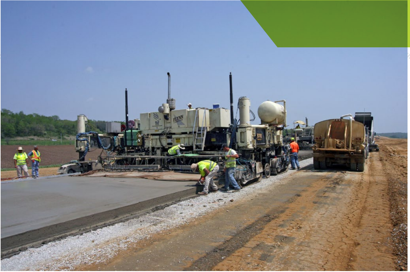
Note the lack of a stringline on the haul road next to the Guntert & Zimmerman paver. Two prisms mounted on masts help position the paver for the robotic total stations.
