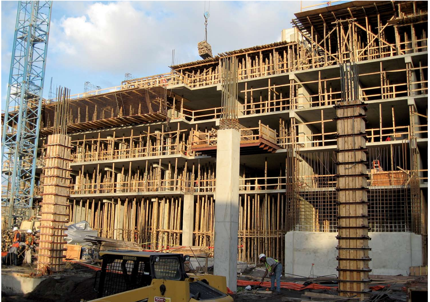
Scanning is increasingly used in construction QA surveys. Image courtesy: JMR Surveying Group, LLC
